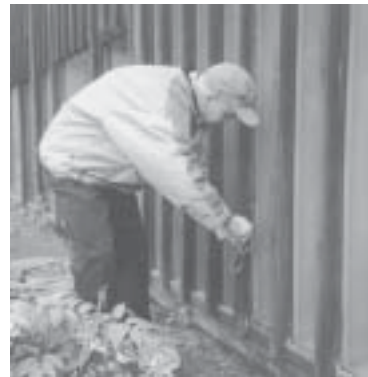
Windows of St. John the Baptist Episcopal Church are caulked as part of the congregation's pledge to conserve energy.
